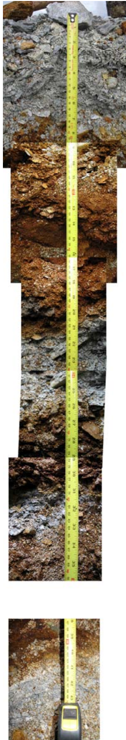
Five-Year-Uncovered Crib – Vertical Profile in the Trench to a Depth of 1.10 m.
